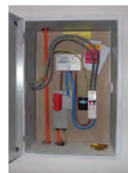
▶ An example of a suitably enclosed meter cupboard
